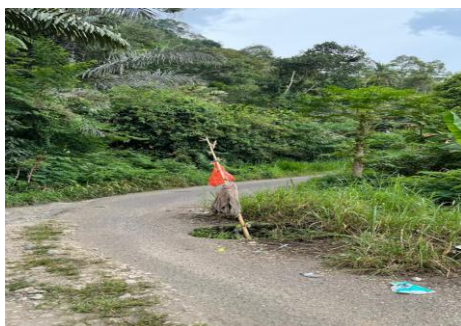
Fig. 4. Roadside hole during daytime.
