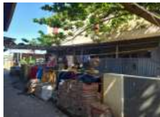
The condition of the building is not in accordance with the standard
