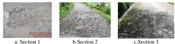
Figure 1. Road Surface Conditions Observed
