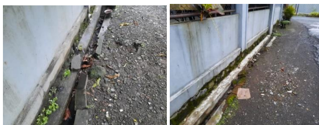
Fig. 2. The initial condition of drainage in Poharin housing complex
