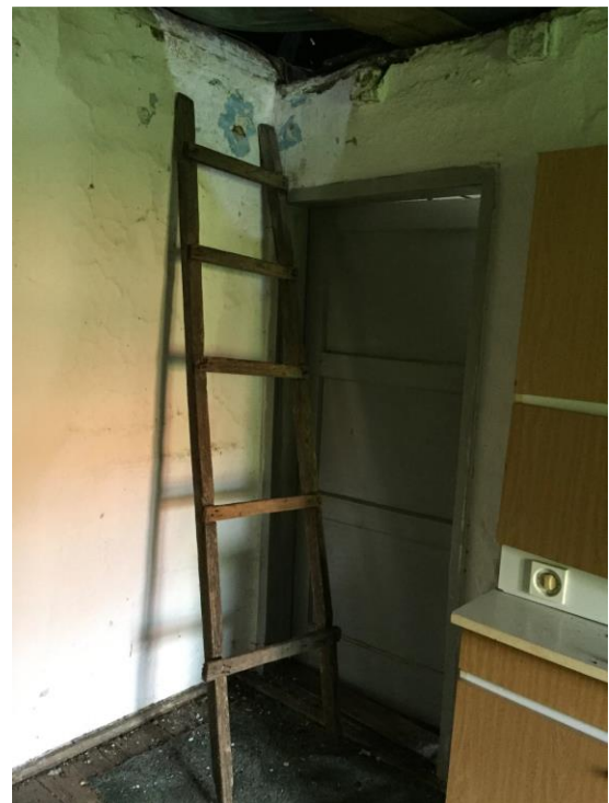
Figure 11. Ladder to exit the proctor attic. Although portable, the ladder was constantly in place due to the frequent communication between the “kuća” and the attic
