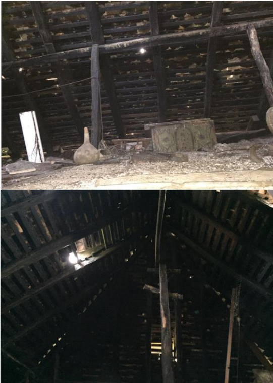
Figure 12. The attic space is open, with an engineered roof construction Source: Author (7/27/2016)
