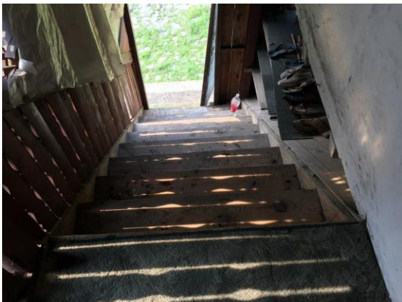
Figure 9. Wooden staircase which leads from the outside to the divanhana, ie to the residential floor on the first floor
