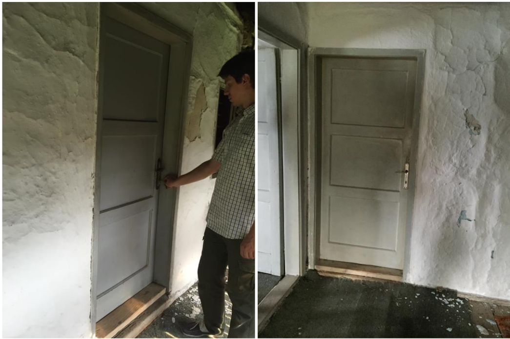
Figure 27. Entrance door to the residential floor, on the first floor (left) and the door on the veranda (right). The door was designed and made in the 70s of the 20th century.
