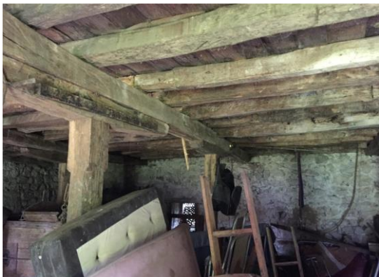
Figure 13. Ground floor - first floor structure visible from the ground floor space Source: Author (7/27/2016)
