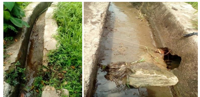
Fig. 1. The condition of irrigation channel in Lokoliku
