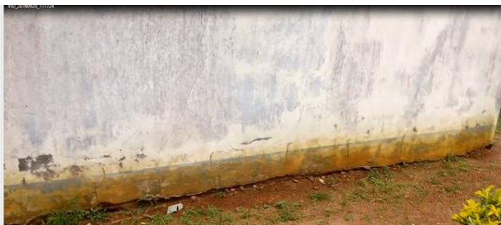
Video Showing the Affected Part of the Deans Office S.E.S
