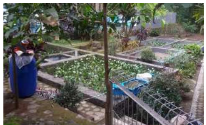
Fig. 1. The condition of communal wastewater plant (IPAL) Tlogomas Malang
