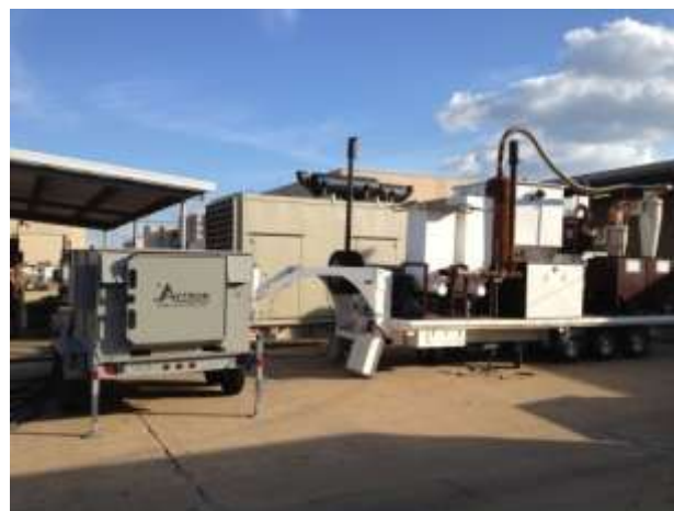
Fig. 4. The mobile gasifier power testing showing load bank on the foreground
