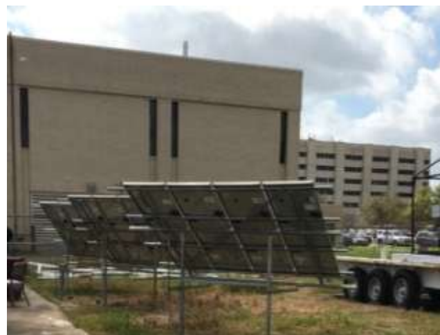
Fig. 3. Photo of the new CdTe 3 kW solar pV system at AERL complex
